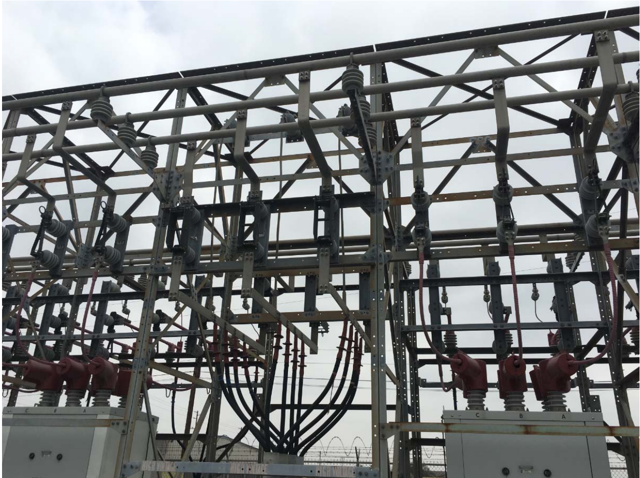
Picture 3: Existing adjacent switchrack, closeup looking south
