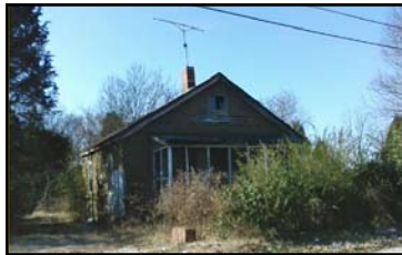
Sub-standard housing and overgrown vegetation
